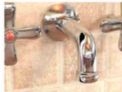
All plumbing & bathroom pipes
